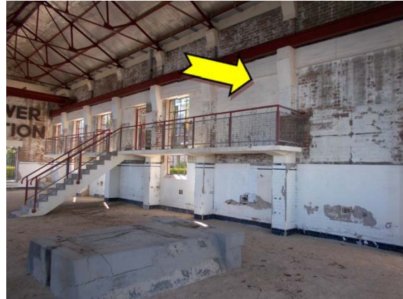
Photo 2. Interior, throughout, walls – suspected lead-containing white upper paint systems.
